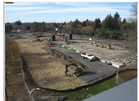
SOURCE: CLACKAMAS COMMUNITY COLLEGE - The demolition and abatement is completed now, and the webcam on the construction site is available here: dwpwebcams.com/ccc/
